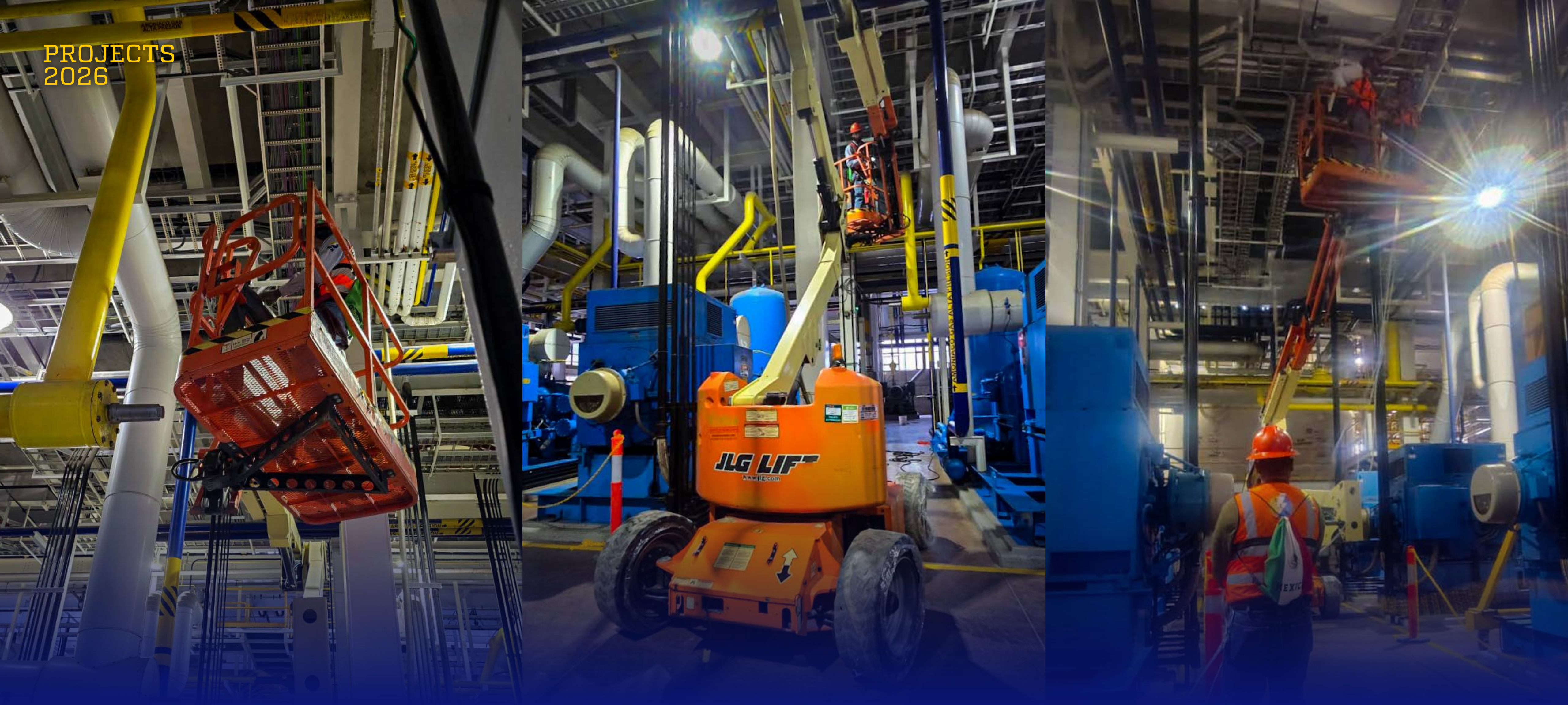
Installation of an ammonia detection system with an alarm and warning lights to enhance operational safety in the area.
